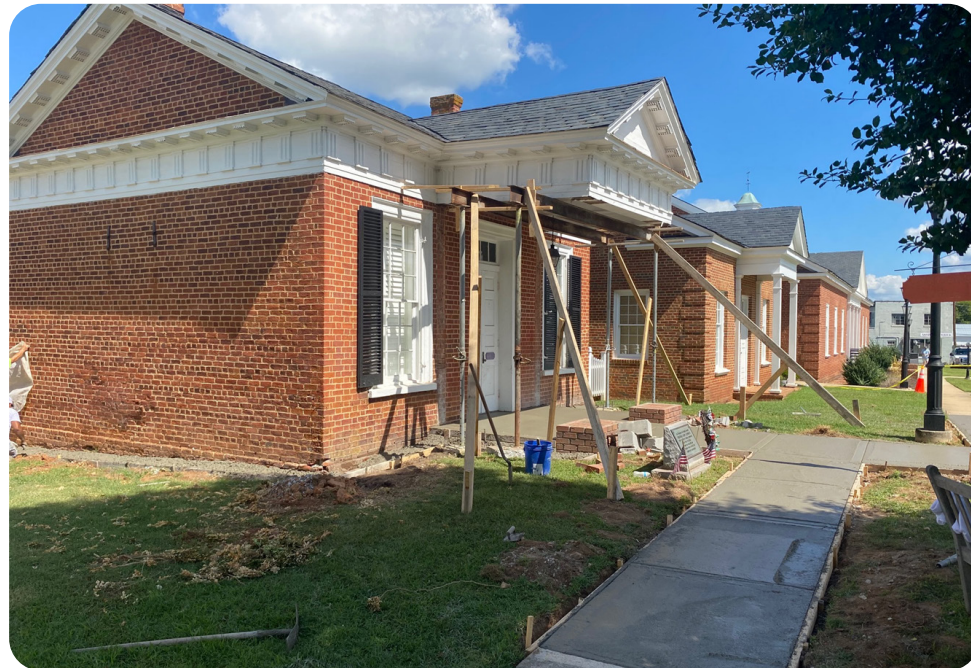
The Capital Improvement funding assists with critical projects, such as the restoration of Cumberland's historic court house facilities.
