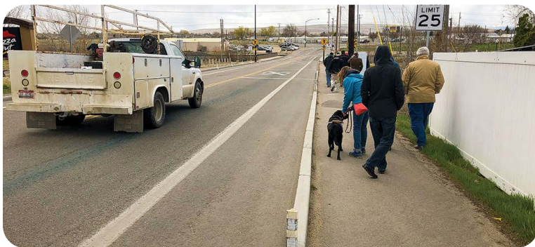
Extruded curb treatments, like these in Kuna, Idaho, are used in other rural areas to create safe pedestrian walkways without the full cost of sidewalks. Photo by Don Kostelec, APA
